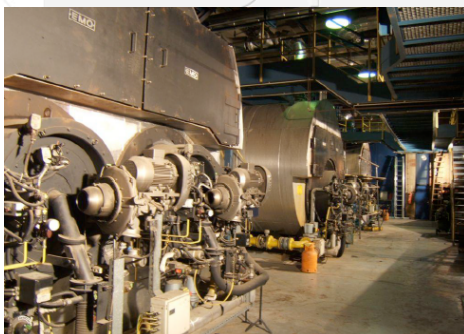
Hot water gas boilers rated at 18.5 MW 17.4 MW and 9.2 MW before replacing
